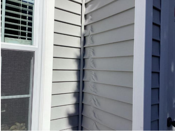
Vinyl siding warp at fire control panel room
