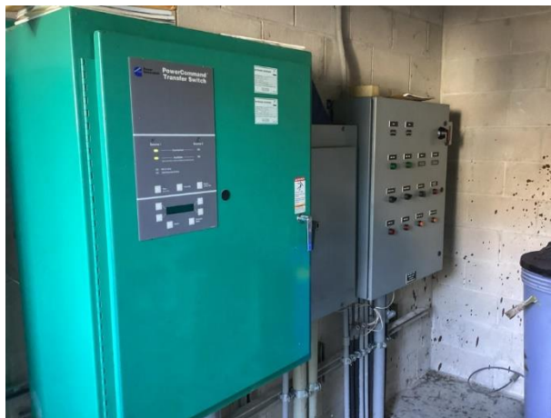
Lift station controls overview
