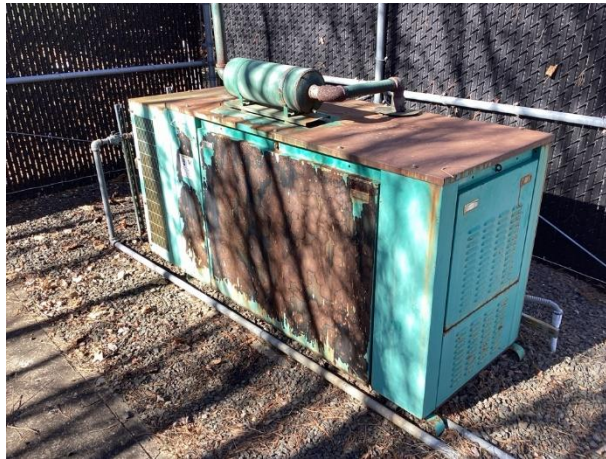
Generator overview (note: significant rust)
