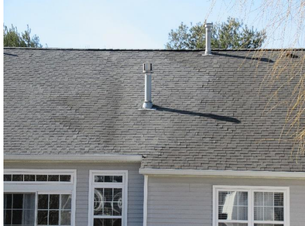
General asphalt shingle deterioration
