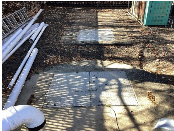
Lift station pumps located under manhole cover
