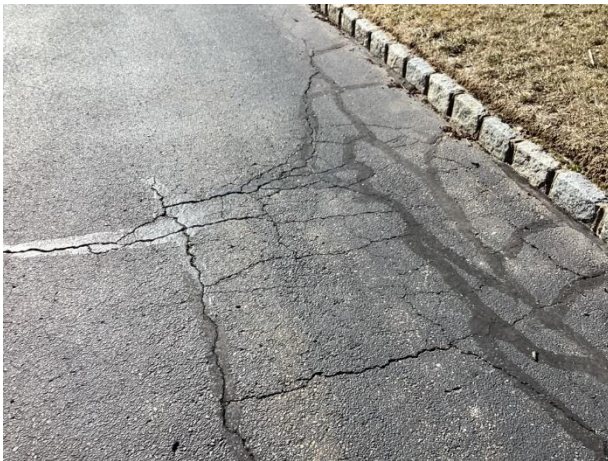
Cracks and previous repairs at street
