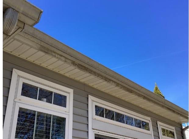
Stains due to undersized gutters
