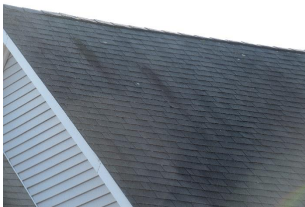
Asphalt shingle stains
