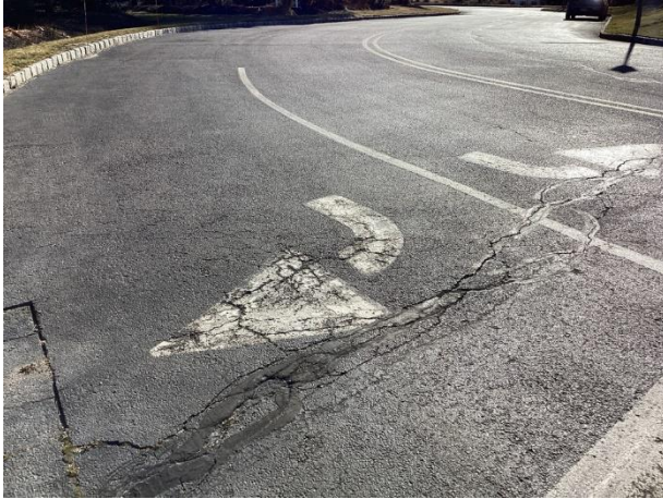
Cracks at property entrance
