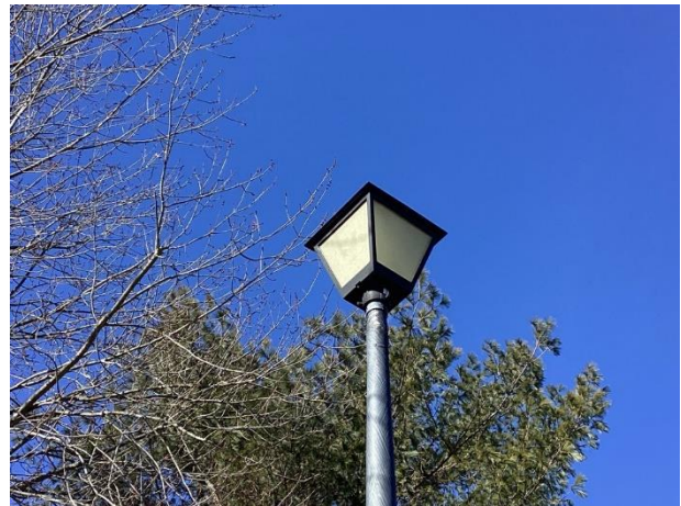
Typical light fixture overview
