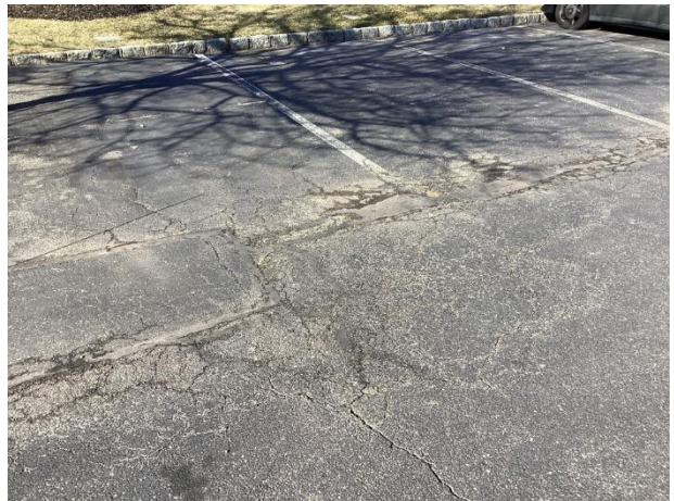
Cracks, stains and general deterioration at parking area
