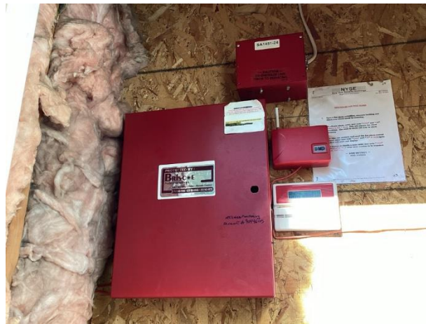
Typical control panel overview
