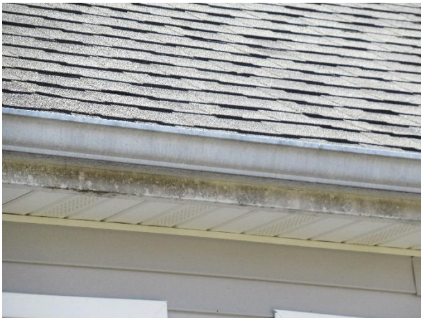
Stains due to undersized gutters
