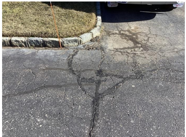
Cracks and previous repairs at parking area
