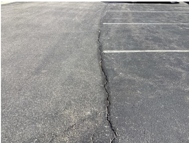
Crack between street and parking area
