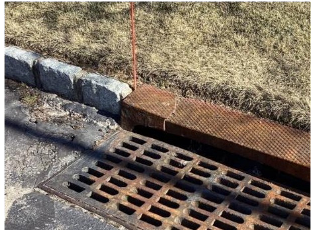
Damage by unit 28
