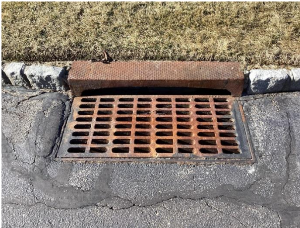
Previous repairs around catch basin
