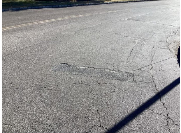
Cracks at property entrance
