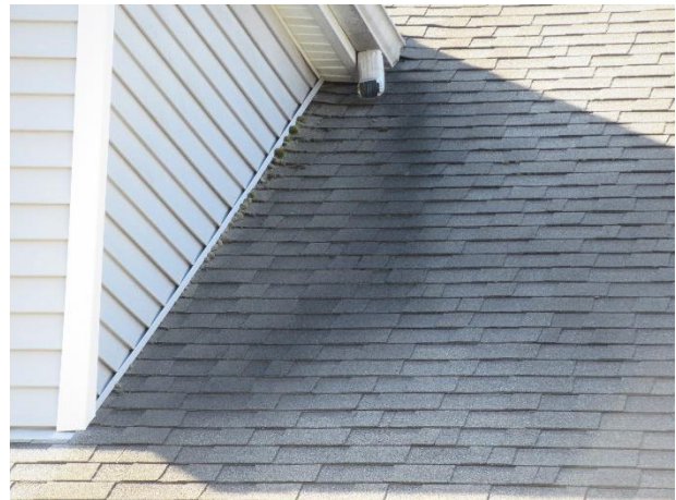
Example of downspout discharging water directly onto lower roof
